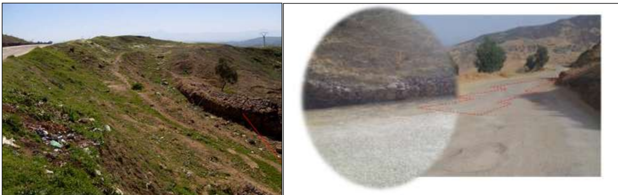
Figure 2: Field photographs showing surface disorders and slope deformation along the affected road section.
