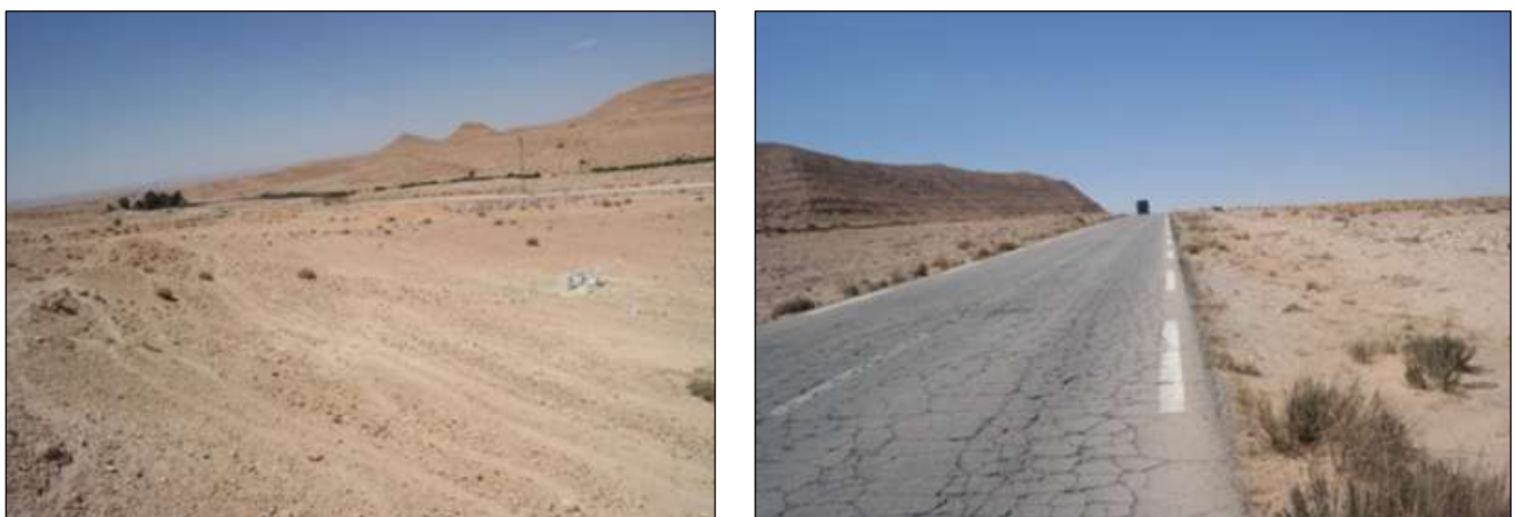
Figure 2: Natural ravines and collapses in RN89: PK 28+500.
