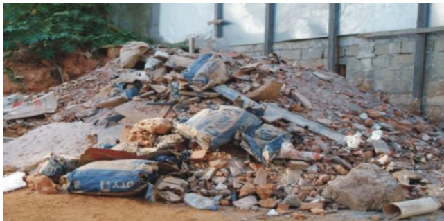
Figure 2 - Incorrect Waste Disposal. Source: [15].
