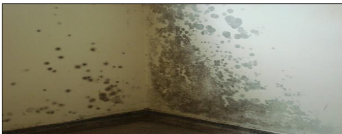
Figure 4: Wall mold caused by moisture. Source: Authors, (2020).
