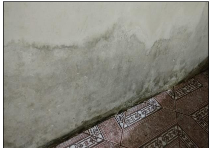
Figure 1: Wall with pathology caused by capillarity.
