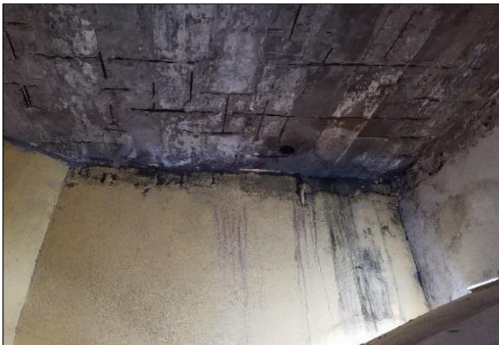
Figure 2: Infiltration in reinforced concrete slab. Source: Authors, (2020).
