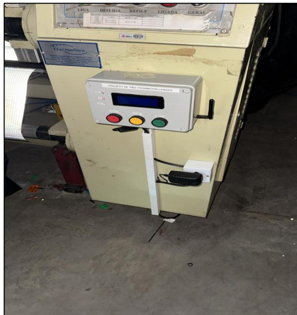
Figure 6: Collector Installed on the Machine.
