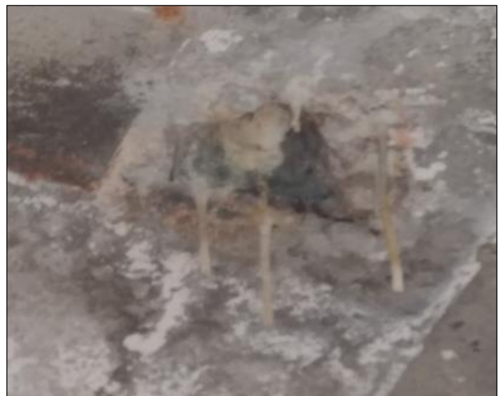
Figure 5: Efflorescence and leaching in the semi-open hole in the service area slab. Source: Authors, (2020).
