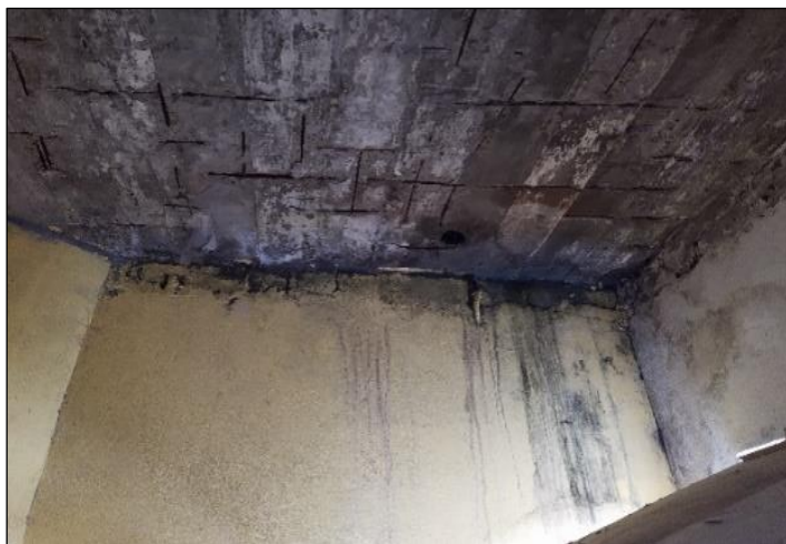
Figure 2: Infiltration in reinforced concrete slab. Source: Authors, (2020).
