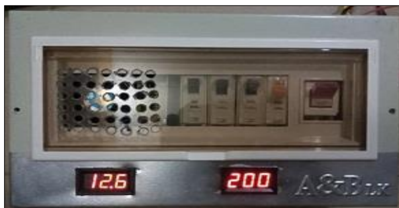
Figure 4: Constructed Hybrid Distribution Board Powered. Source: Authors, (2021).
