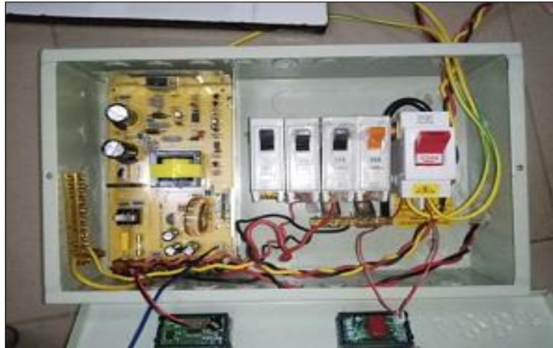
Figure 2: Internal Connection when all cables are connected. Source: Authors, (2021).
