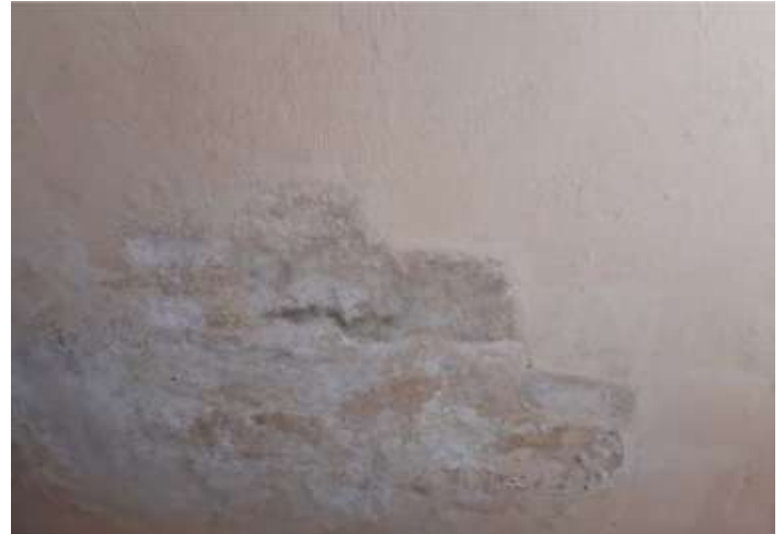
Figure 3: Appearance of efflorescence on the masonry wall. Source: Authors, (2025).
