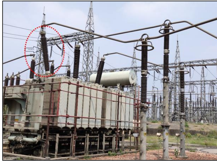
Figure 1: Site photo depicting tilted R-phase failed HV transformer bushing. Source: Author, (2026).
