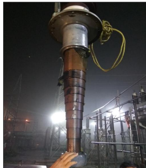
Figure 3: Site photo depicting tilted R-phase failed HV transformer bushing. Source: Author, (2026).
