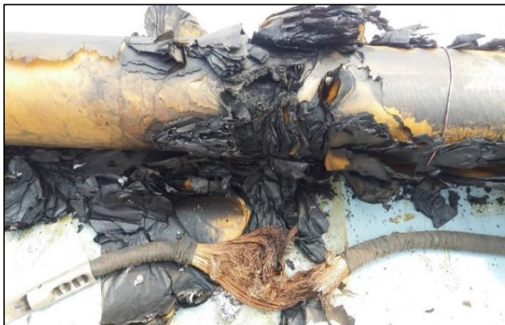
Figure 2: Failed 245 kV Condenser bushing with displaying a failed Draw Lead in the bottom of the picture. Source: Author, (2026).
